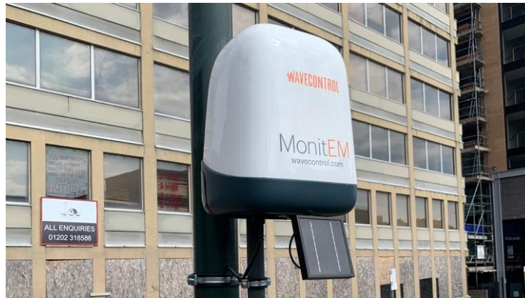
An electromagnet Field (EMF) monitor continually monitoring emissions from our 5G and other wireless installations
